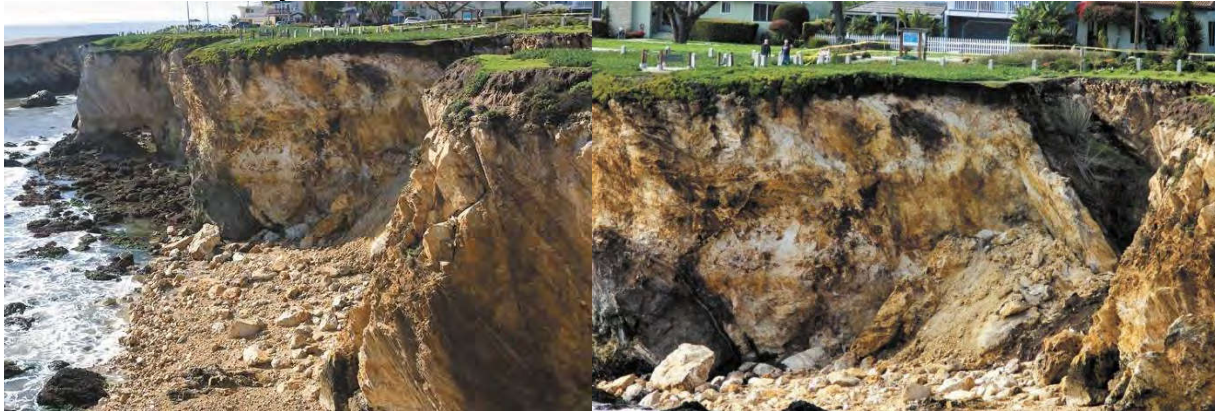
Figure 5-33 Bluff Erosion and Overlying Development at Dinosaur Caves Park in Pismo Beach, January 2010
