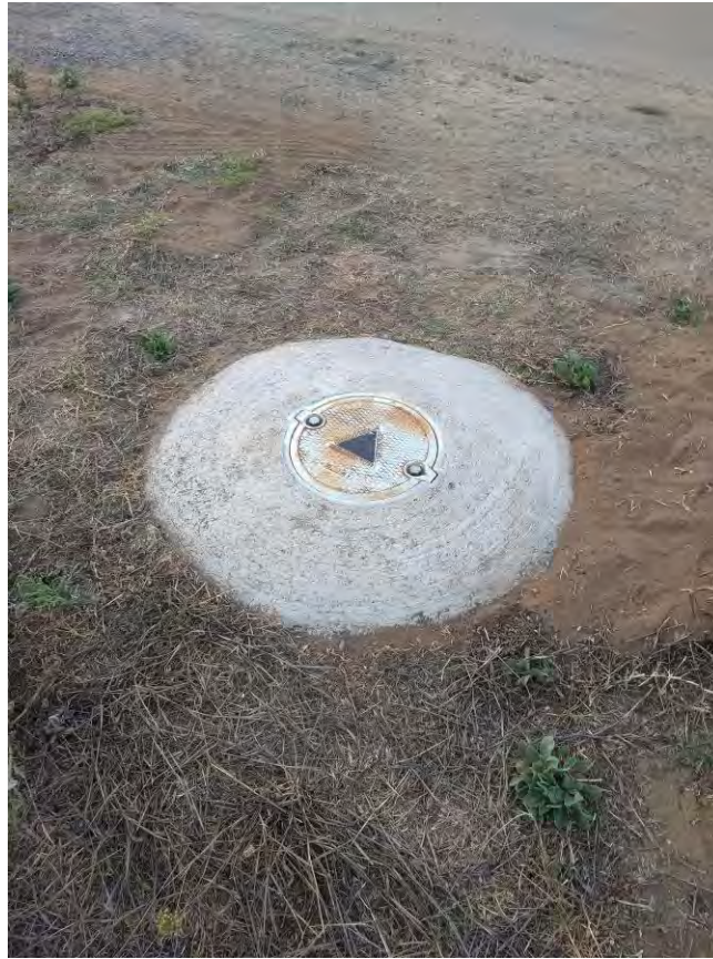
Figure 1. Typical 12-inch monitoring well box
